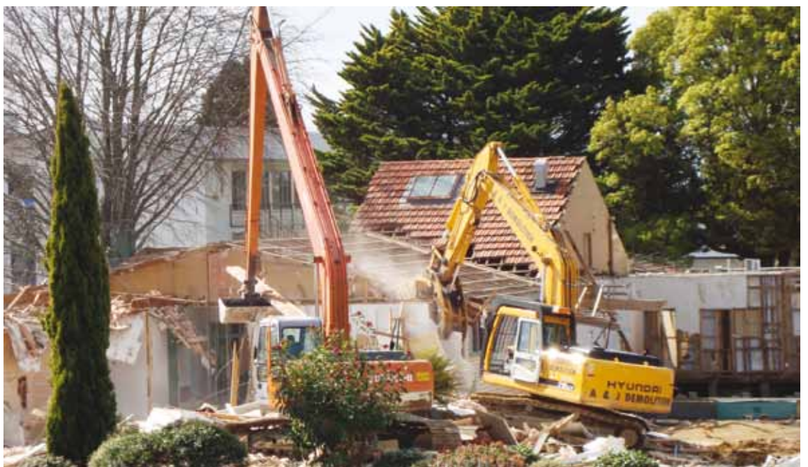
The last walls of Tauranga Hospital's former maternity unit came down in early September to make way for a new 132-space visitor car park.
