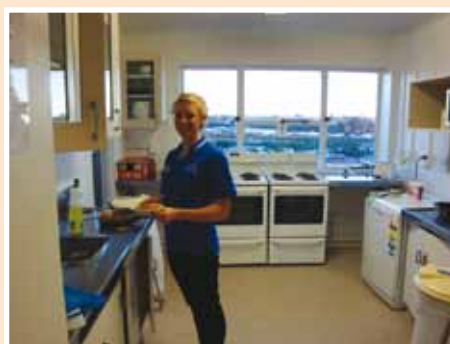
The Jacaranda House kitchen upgrade included installation of a pantry, additional oven, new fridges and a dishwasher.
